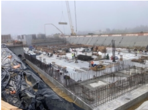
Pure Water Facility
