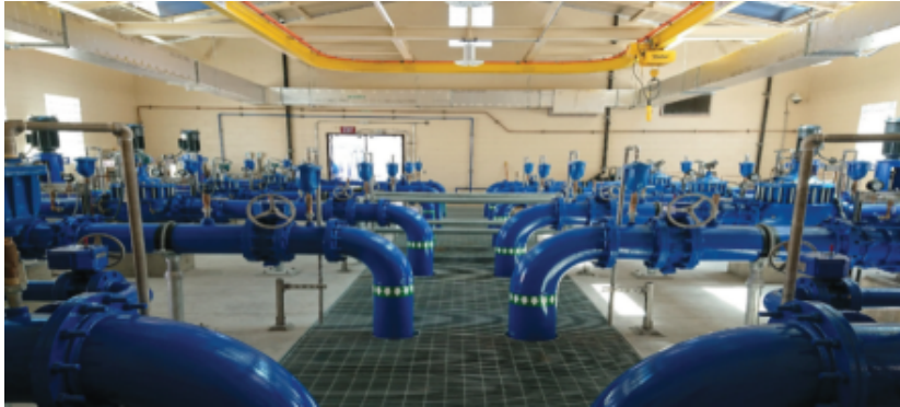
Tierrasanta Pump station
