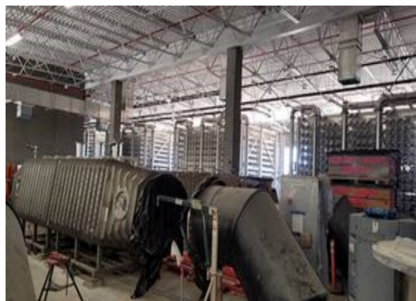
UV Reactors and Reverse Osmosis Equipment in Background
