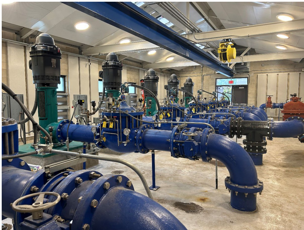
Inside 69 th and Mohawk Pump Station, winner of APWA Project of the Year Award for Utilities.
